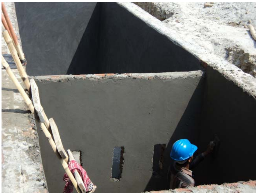
Photo No.2: Construction work of septic tank of Mosque at Bakharakandi RS5
