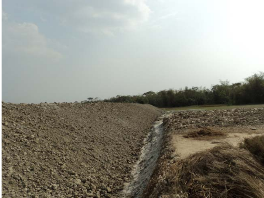
Photo No. 1: Top soil cladding of side slope at Service Area- 3, Kutubpur
